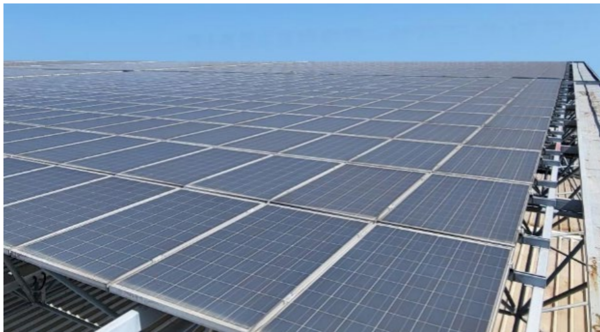
Fii Distributed Photovoltaic Power Generation System
